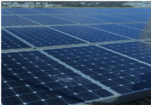
Solar PV modules installed on the Guildhall
